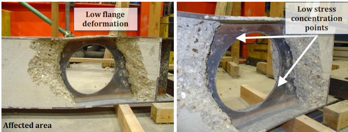
Fig. 14: Failure mode for partially encased USFB No.2 at opening after removal of the damaged concrete
