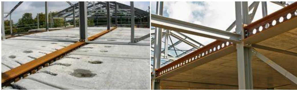
Fig. 1: USFB used with profiled steel decking (top) and with precast concrete unit (bottom) (adopted by [8])
